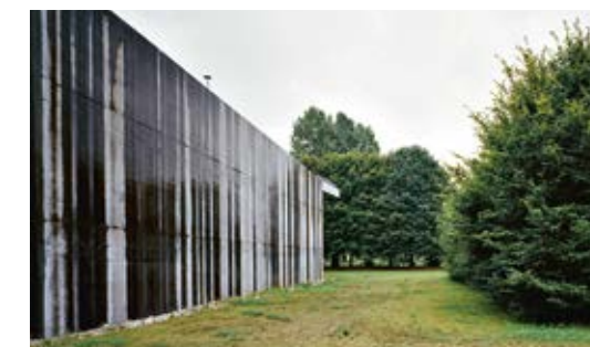
Concrete end walls with pattern created by the rain.
